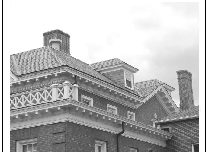
This shows the rebuilt chimney on the left, and repointed one on the right, and many replaced dentils under the roof edges.
